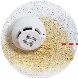
Stains on interior ceilings and walls or mold and mildew growth Possible causes: Inadequate or faulty shingle underlayment allowing leakage; inadequate ventilation
