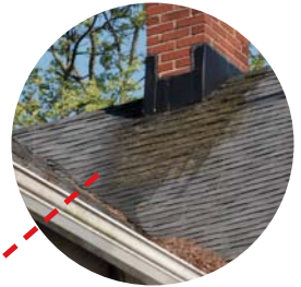
Dark, "dirty-looking" areas on your roof Possible causes: Loss of granules due to age of shingles or blue-green algae stains
