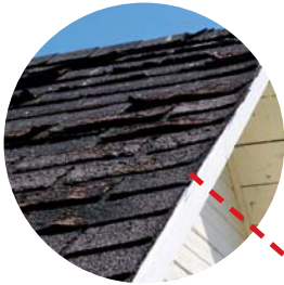
Missing, cracked, or curling shingles Possible cause: Shingles have reached the end of their useful life
