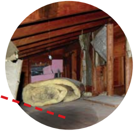
Leakage in attic after driving rain Possible causes: Degraded or inadequate shingle underlayment; deteriorated flashing
