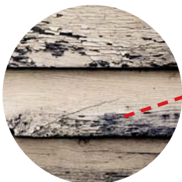
Blistering and/or peeling of outside paint Possible cause: Excessive moisture or high humidity due to poor attic ventilation
