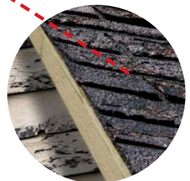
Roof shingle, sheathing, and siding decay Possible cause: Poor attic ventilation
